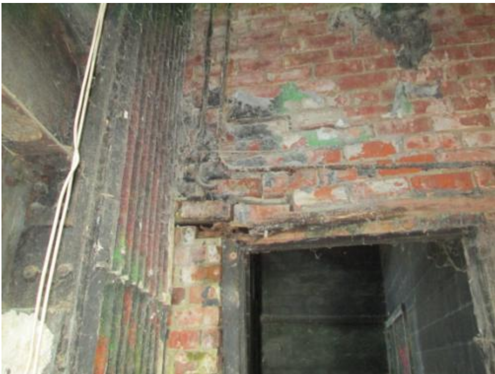
Photograph 64 – Failed timber lintel above end door opening to lean-to
