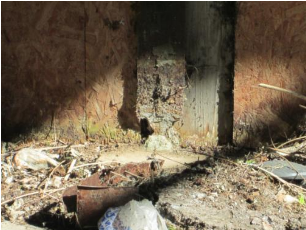
Photograph 68 – Rusting column to rear elevation (worst case)
