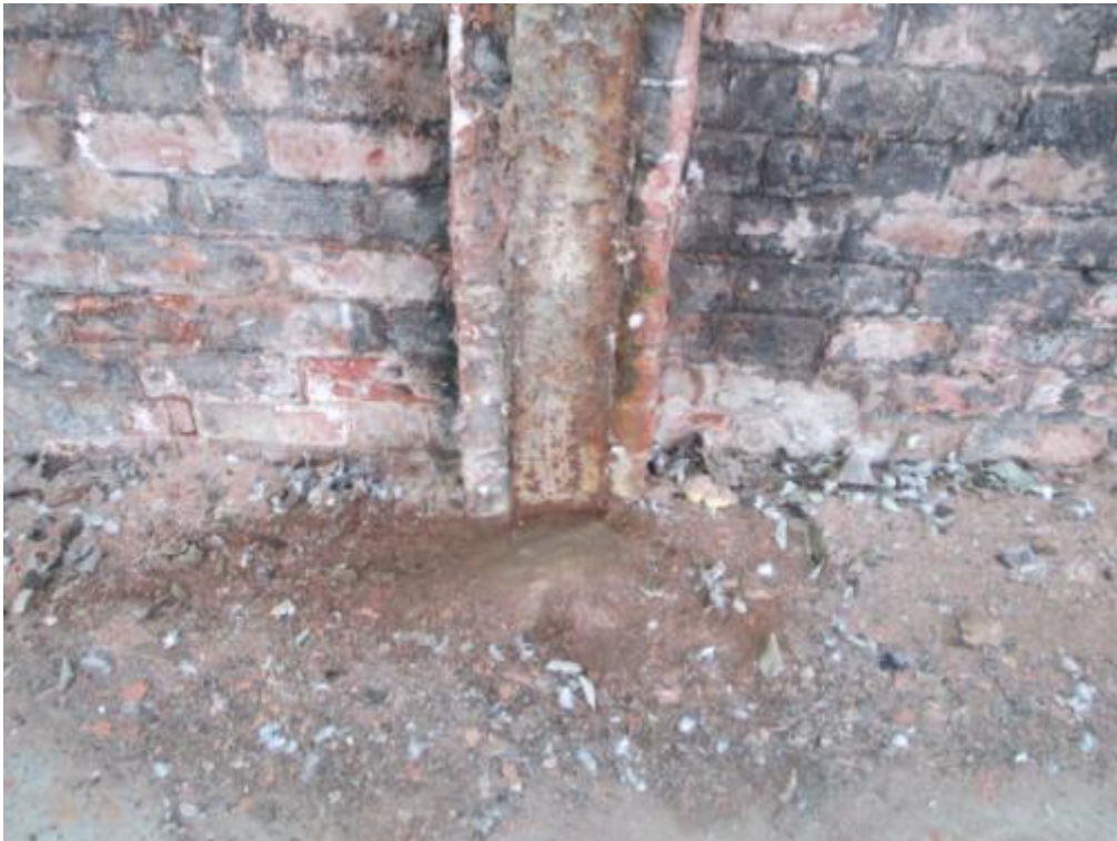
Photograph 70 – Typical view of rusting column to front elevation
