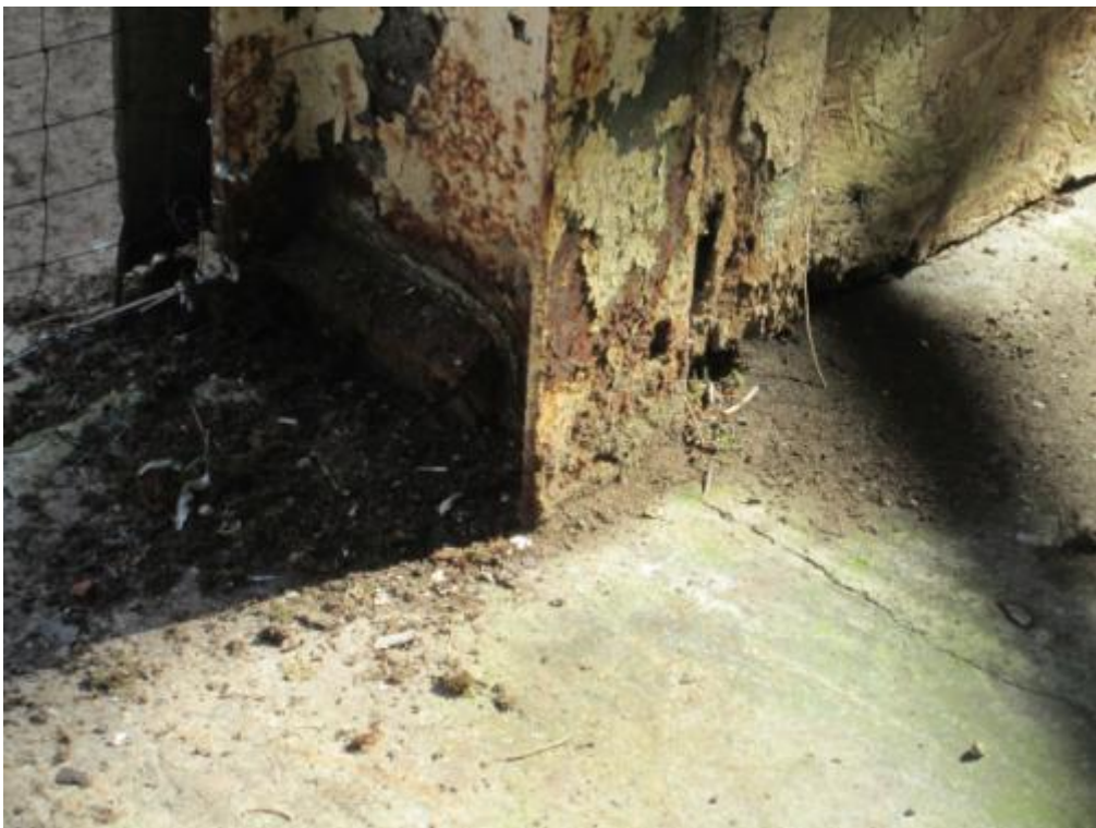
Photograph 69 – Typical view of rusting column to rear elevation
